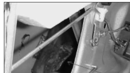
Pad Incorrectly Installed
