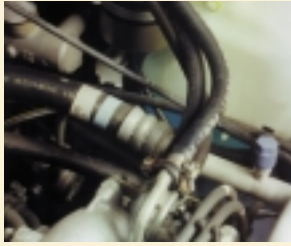
Fuel Filters and Hoses
